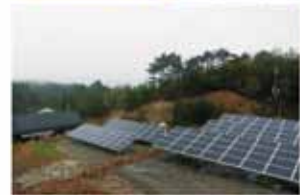
Ground Solar Power Plant Nara Prefecture, Japan 66kW Jun 2016
