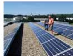
Stuttgart, Germany 400kW 2011
