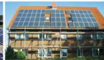
Warnow, Germany 20kW 2011
