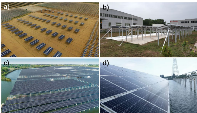
Figure 7 (a) China Kubuqi 336kWp project using bifacial module and oblique uniaxial tracker; b) TÜV SÜD's bifacial field test project in Hainan, China; c)&d) The Chinese Sihong "Top Runner" project using nearly 275MWp Hi-MO3 modules
